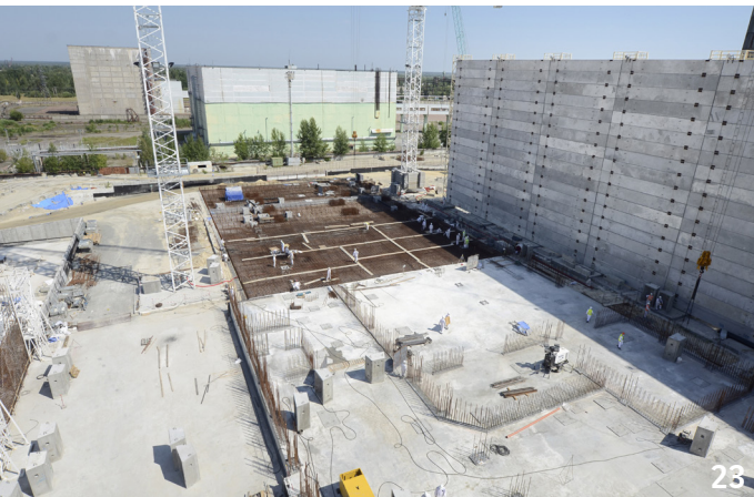
April 2014: First concrete poured for the foundations of the Technological Building and auxiliary buildings. - ©Francis Vigouroux
