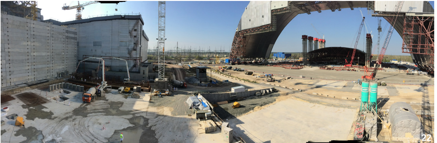
April 2014: First concrete poured for the foundations of the Technological Building and auxiliary buildings. - ©Francis Vigouroux
