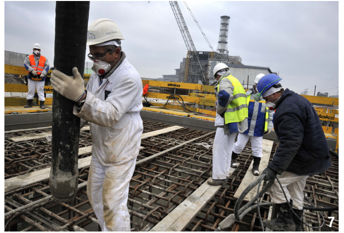
7 September 2011: Installation of the longitudinal beams in the assembly area. - @Francis Vigouroux
