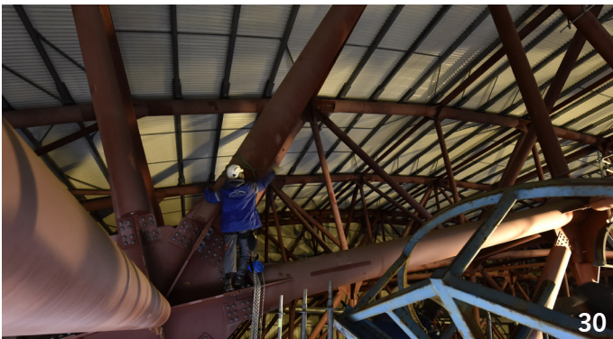
June 2015: Work starts on the electrical and ventilation systems inside the arch. - ©Francis Vigouroux
