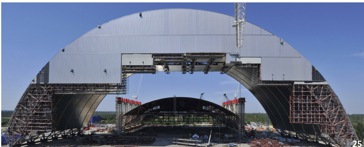
August 2014: Second lifting operation for the second half of the arch. - ©Francis Vigouroux
