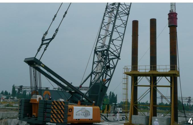
4 August 2010: Driving the metal piles for the longitudinal beams in the assembly area.
