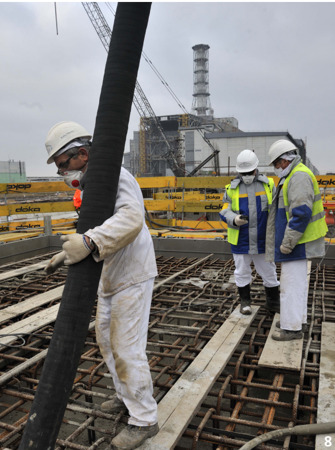
8 September 2011: Installation of the longitudinal beams in the assembly area. - @Francis Vigouroux
