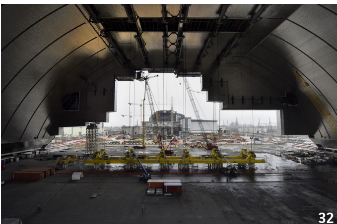
November 2015: Lifting the first overhead bridge cranes inside the arch. ©Francis Vigouroux
