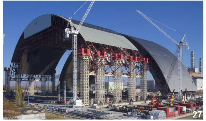
October 2014: Third and final lifting operation for the second half of the arch.
