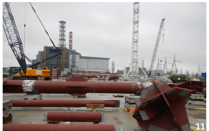
11 April 2012: Delivery of the first arch components on site and start on the frame assembly.
