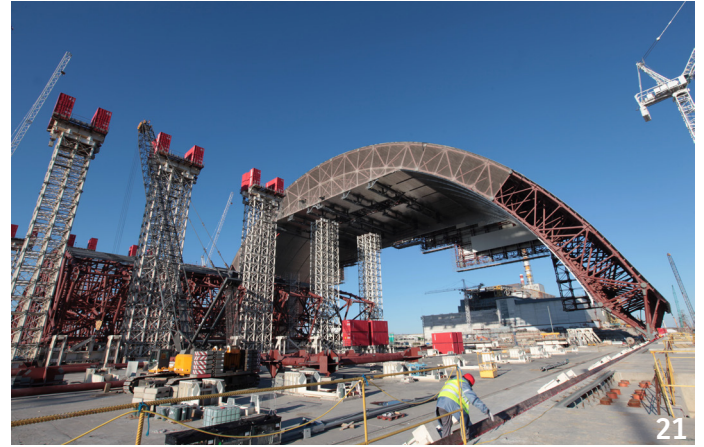
April 2014: First half of the arch pushed to the waiting position (4) and first lifting operation for the second half.
